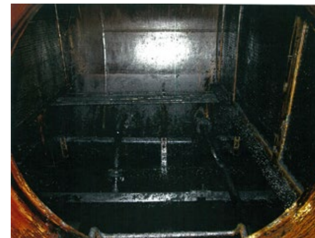
Fig.3 Inside of a desalter with large amounts of buildup
